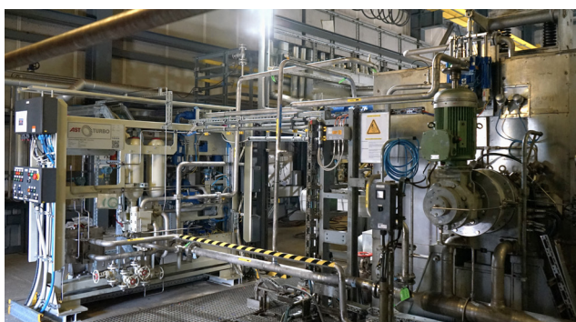
Figure 2. Rack integrated into existing compression train.
