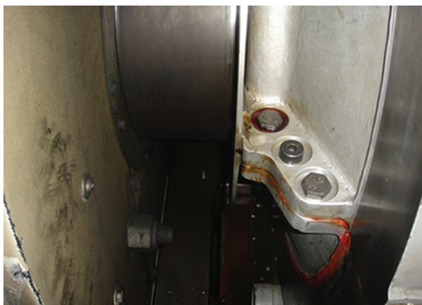
Figure 2. Reoccurring failure can be avoided: oil leak through oil deflector horizontal joint.
